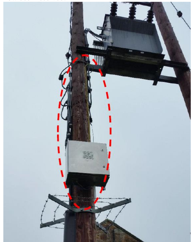
Fig. 24: Receiving station 1 mounted on OHL pole
