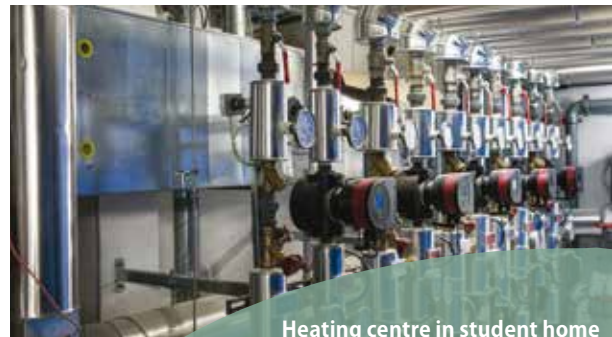
Heating centre in student home
